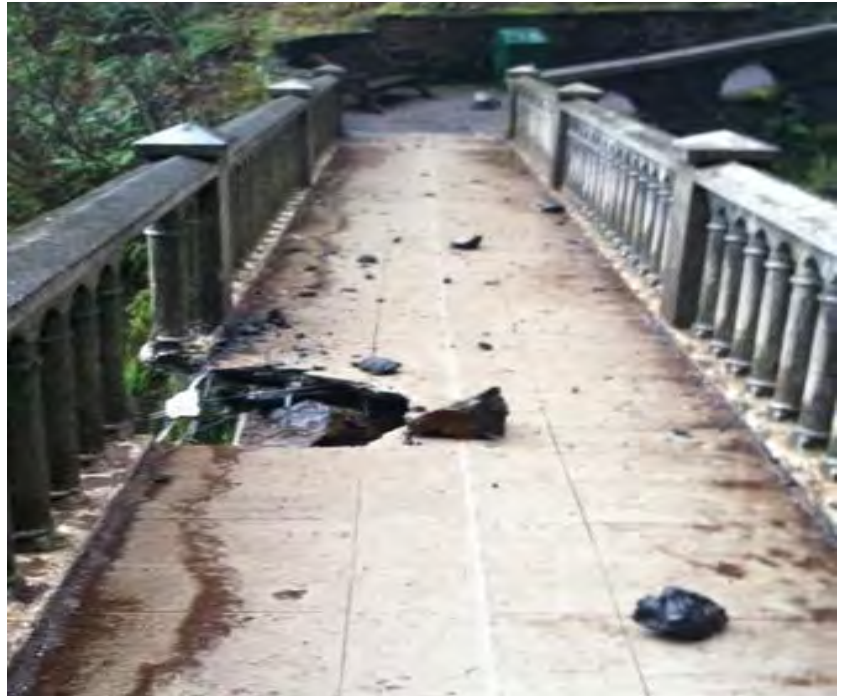
2014 rock fall creating hole in Benson Bridge walkway
