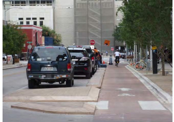
Figure 8. Concrete island doweled in to roadway to create a protected bicycle lane in Austin, TX.
