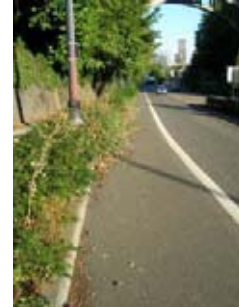
Overgrowth west of Vista Bridge
