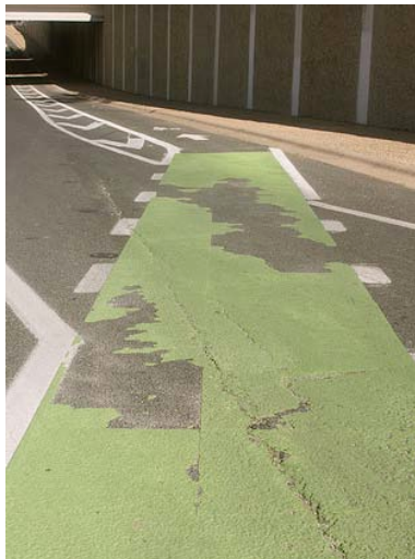
Figure 18. Deteriorating thermoplastic on Dean Keaton Street at one of the I-35 exit ramps (breaking up in sheets)
